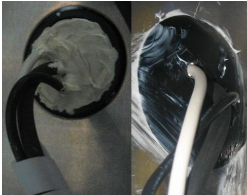
Figure 3.32: Removable sealed cable conduct. It was made from a bathtub plug which was sealed by silicone after the cables were put through.
