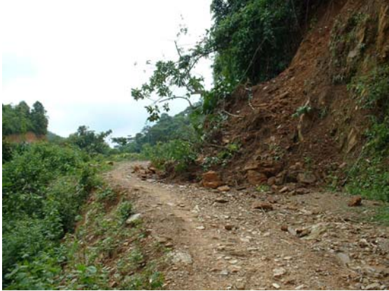
Figure 3: Track to Ot Luong and Ban Dau, blocked by a land slide Rößler (2004)
